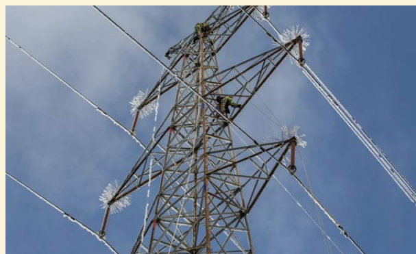
Photo taken on November 20, 2020 shows technicians of State Grid Yanbian Power Supply Company repairing power supply lines in Dunhua of Yanbian Korean Autonomous Prefecture, Northeast China's Jilin Province. Photo: Xinhua
